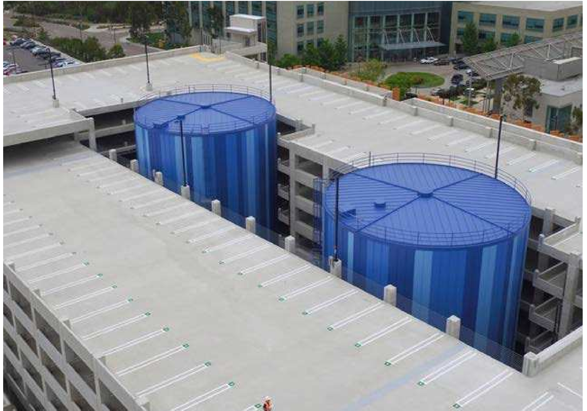
UC San Diego Thermal Storage Tanks
